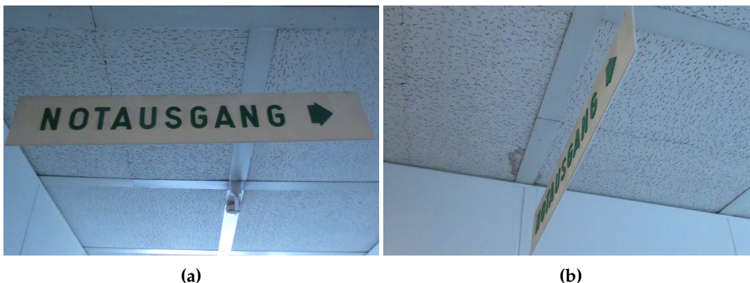
Figure 4.9: Photograph of emergency exit sign, corresponding with the points shown in Figure 4.8. Notice, that, as opposed to what the 3D data suggest, the sign is actually very flat and mounted by two very thin, strings, almost invisible in the photograph.
