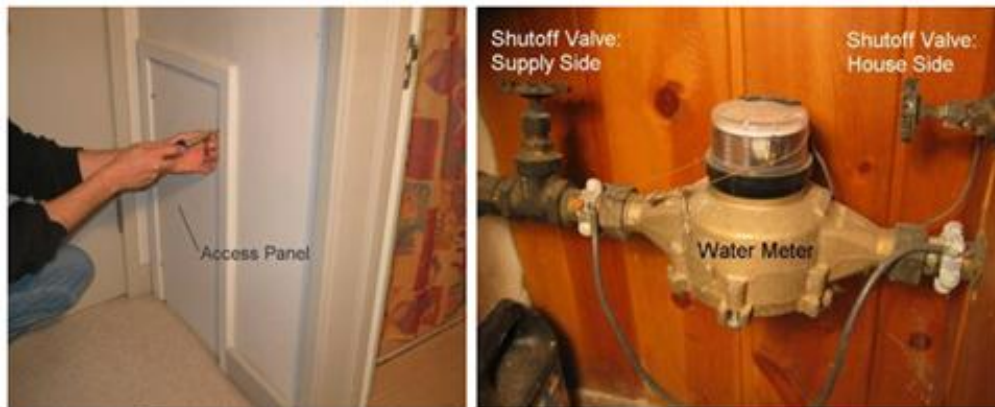
Figure 4.3: Shut-off valve located in access panel inside wall.
